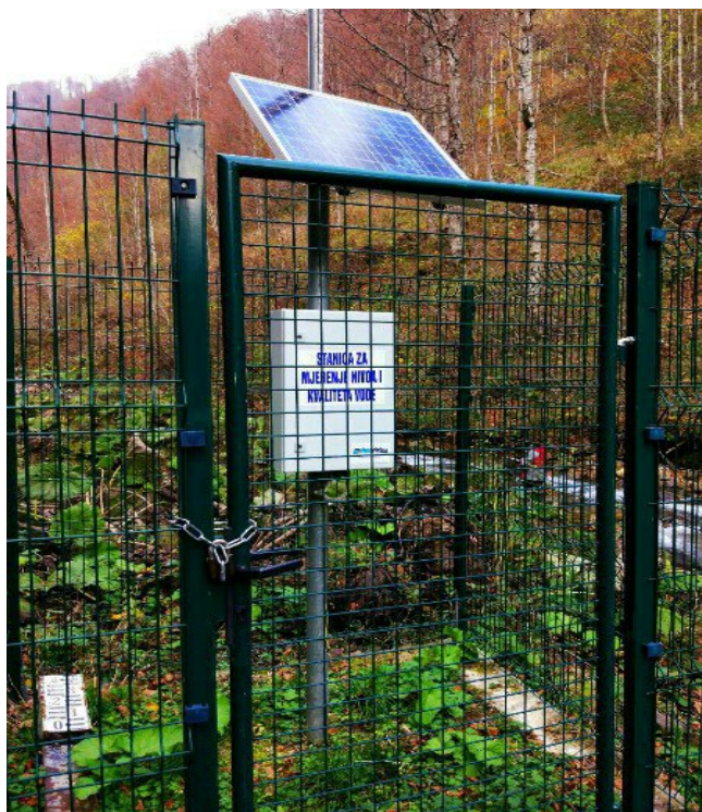
Figure 4a. Automatic hydrological and water quality station at SHPP Podhum 1
